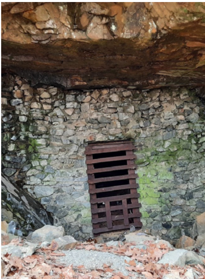
Cranberry Mine entrance with iron plate door at Harriman State Park — Thea Landesberg 2023
